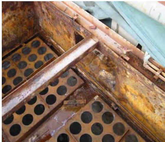
Casing / tube plate corrosion
