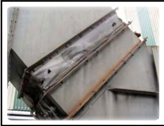
Broken expansion joint
