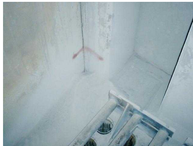
Casing / tube plate leaks
